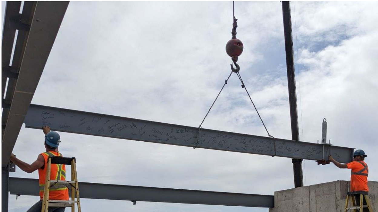
Signed topping off beam for the Delphine and Lloyd Martin Apartments lowered into its final position, June 22, 2023.
